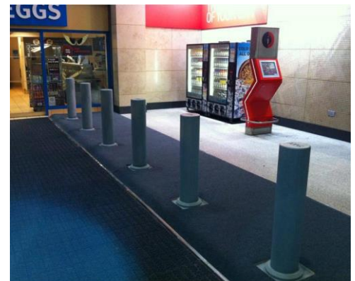
Surface Mounted Bollards Installed Inside a Shopping Centre
